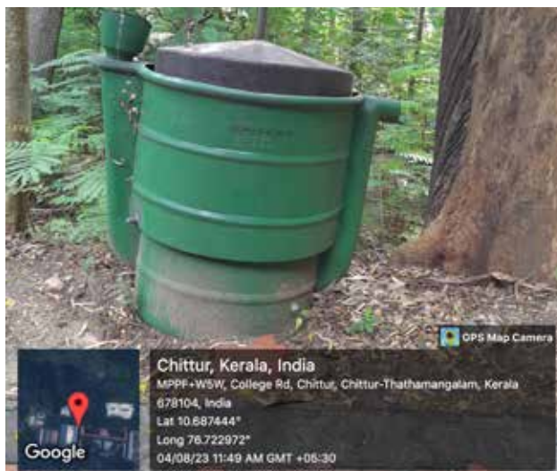
Biogas plant near the canteen which requires maintenance
